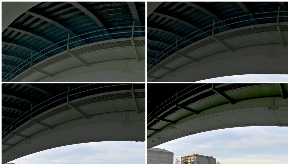
Figure 20: UnderBridgeHigh video sequence tone mapped with the SUB+ZBC technique. Extracted frames 80 (TL), 100 (TR), 120 (BL) and 140 (BR).
